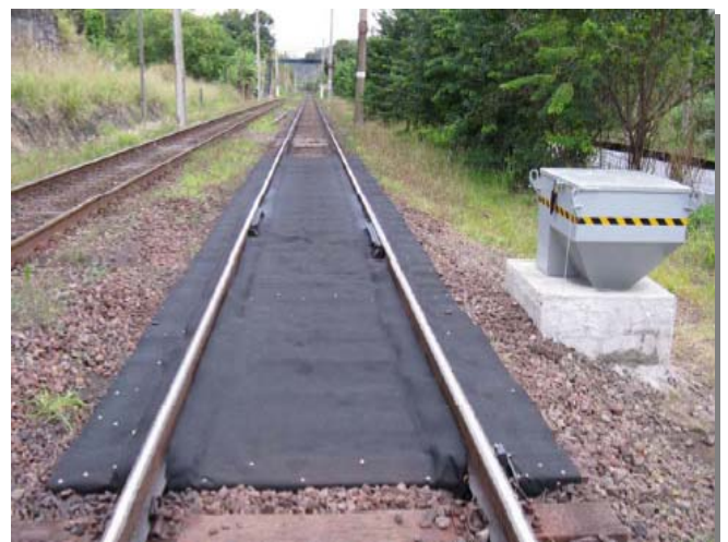
Figure 8 – Wayside lubrication installed in the 2nd test zone (Santana de Barra)
